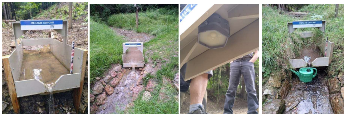
Water measuring stations for measuring flows with online data transmission
